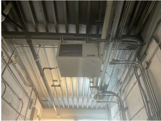
PHOTO #25 NATURAL GAS-FIRED HEATER
