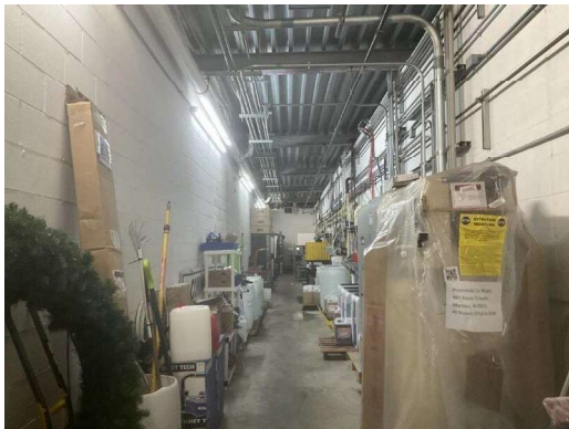
PHOTO #11 CAR WASH EQUIPMENT ROOM
