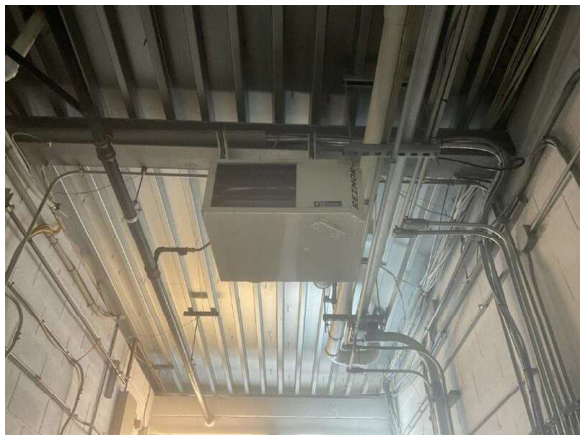
NATURAL GAS-FIRED HEATER
