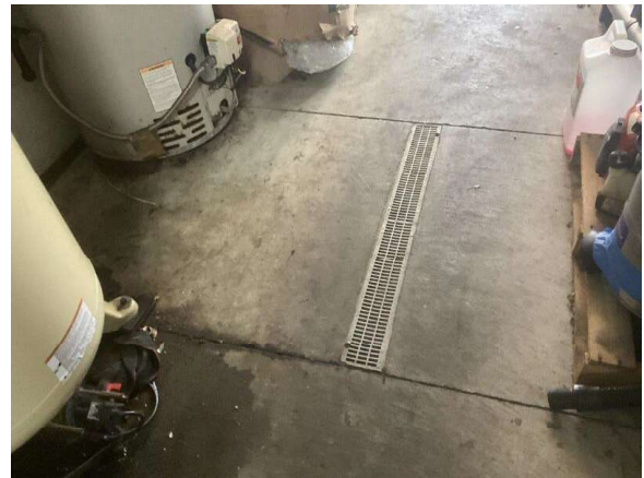
FLOOR TRENCH DRAIN IN EQUIPMENT ROOM
