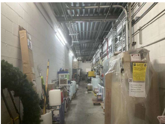
CAR WASH EQUIPMENT ROOM
